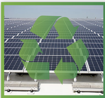
Recycling solar equipment
